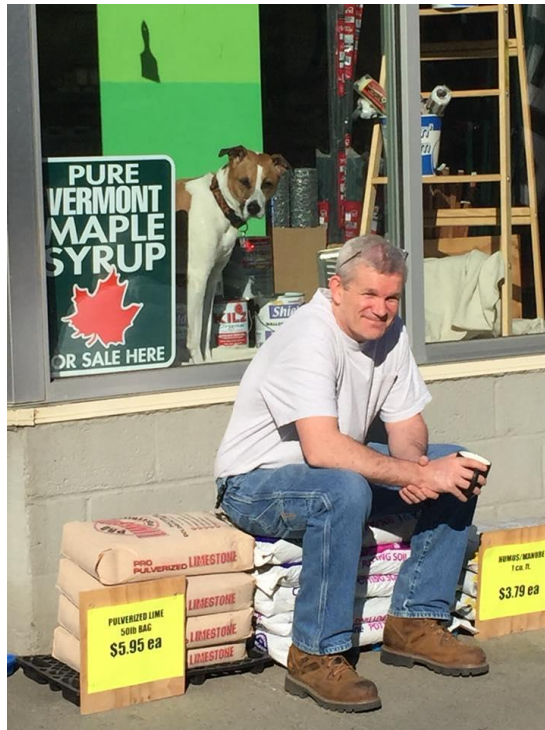
Bethel Resident and Business Owner Brad Andrews and his dog Bunks enjoying a cup of coffee while overlooking a water line repair on Main Street.
